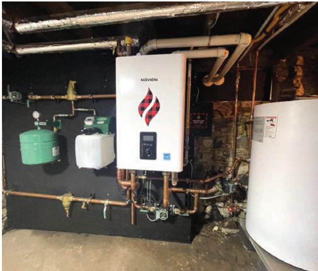
This award-winning residential hydronic system install by Family Tradition Propane Services in Nova Scotia was “simple, serviceable and repeatable,” according to the contest judge.
