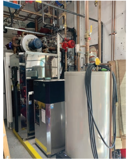
The original single boiler back-up system in the district energy plant was removed for a more efficient and resilient solution.
