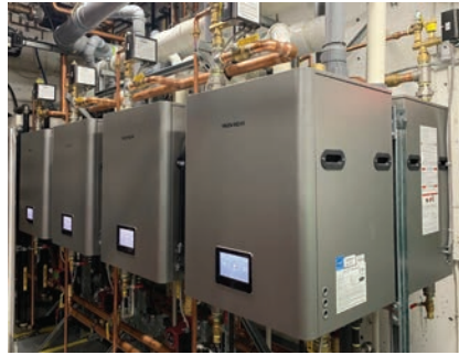
A cascading system of eight boilers provides back-up heating for a geothermal district energy plant in Langford, B.C., installed by South Island Mechanical.
